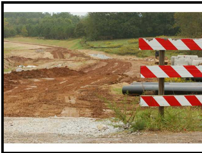
The right of way has been cleared at Plainview Road where Thurmon Tanner Parkway will connect with Mundy Mill Road.
